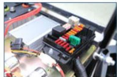
Electric control fuse
